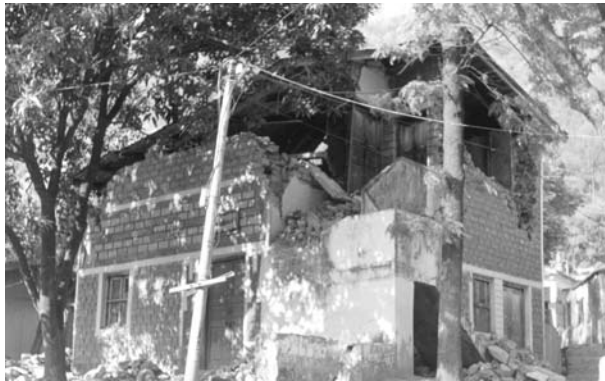
Figure 7.1 : A Damaged Building Due to an Earthquake
