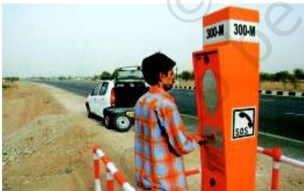
Fig.7.10 : Emergency call box on NH-8
